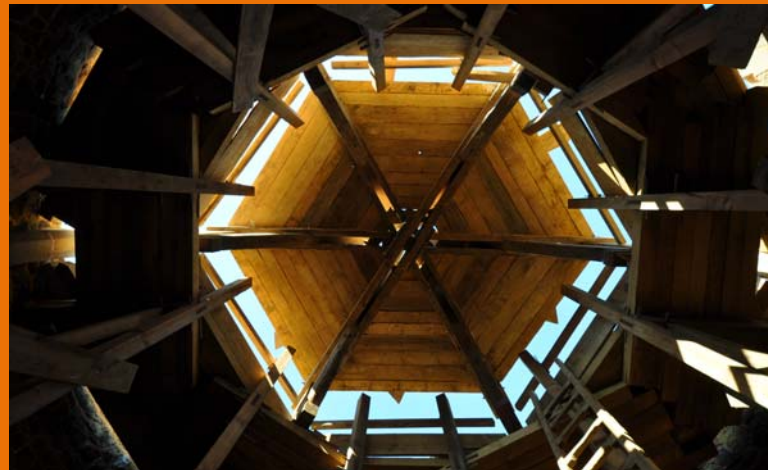
3 November 2010: the centring above the vault seen from below after its installation.
