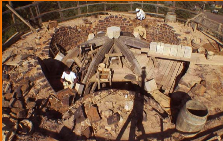
1 August 2011: the wall arches are complete and the keystone has been positioned on the centring.
