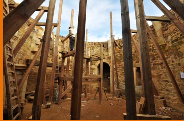
29 August 2010: the carpenters put up the scaffolding which will support the centring.
