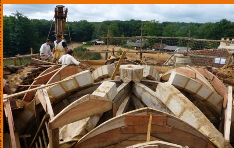
19 August 2011: most of the voussoirs have been positioned on the centring. The counter-keystones are the final voussoirs to be inserted.
