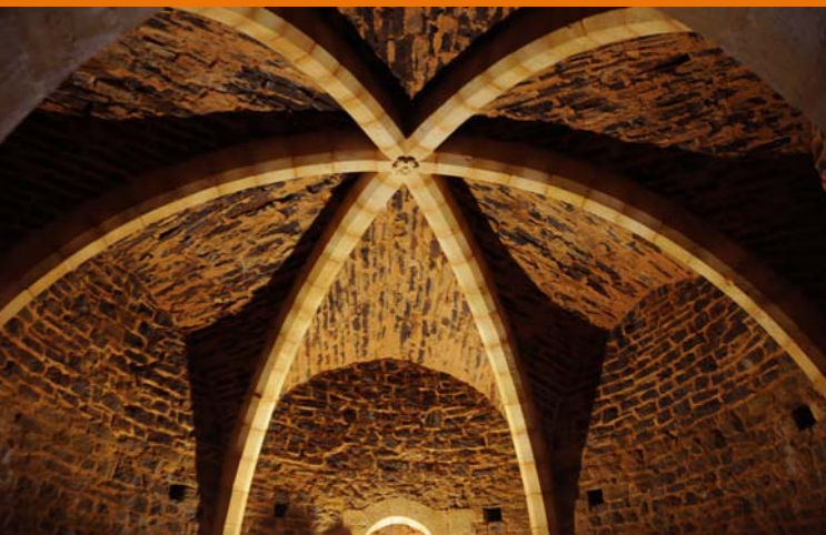
16 October 2011: the scaffolding has been removed and the vault's beauty is revealed for the first time.
