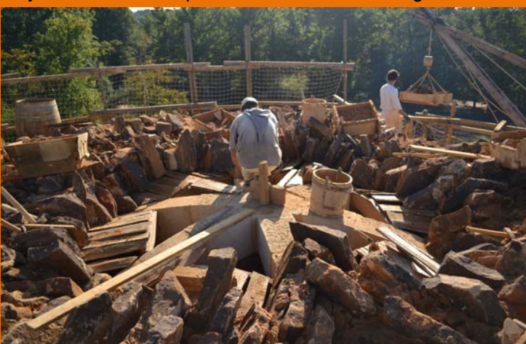
23 September 2011: sandstone flagstones are edge-bedded on wooden shuttering to form the vault's webbing.
