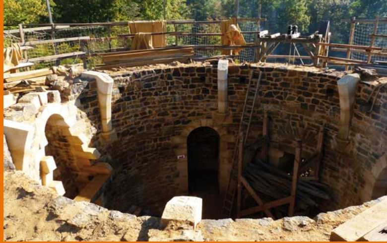
26 August 2010: the exterior walls are up and the 6 corbels and tas-de-charges are in place.
