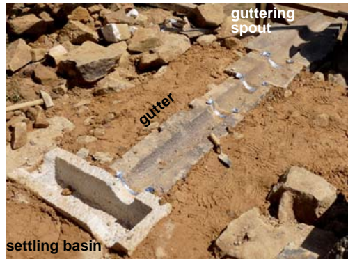
Rainwater drainage system
